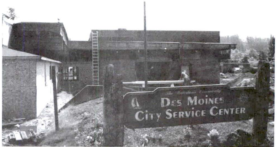
New roofs are being constructed on the existing buildings to blend architecturally with the new building being constructed on the site of the former police station.
